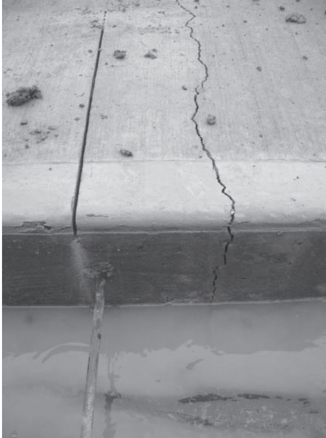
Figure 22.15 Joint cut too shallow.
