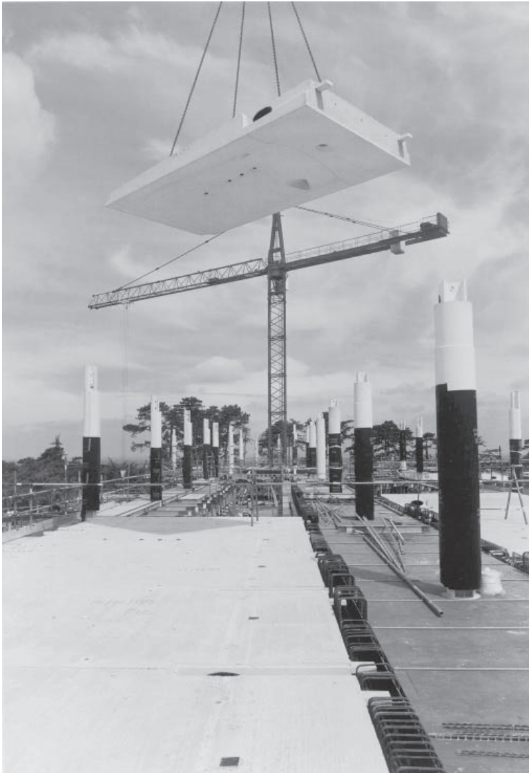
Figure 21.4 Toyota (GB) Ltd, Head Office: Precast concrete two-storey columns and self-finished floor elements combine with in-situ concrete beams and floor topping to enhance the buildability of a cost-effective structure. (Courtesy Takaneka (UK) Ltd and Trent Concrete Ltd.)
