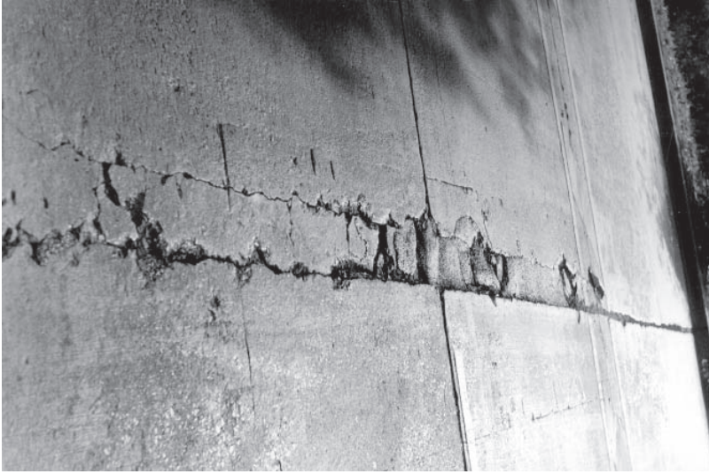
Figure 22.18 Badly bonded tie bars.
