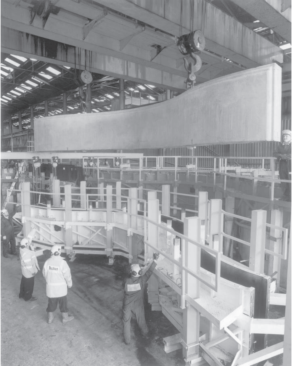
Figure 21.6 Gatwick Airport: Acoustic wall. Stripping a freshly cast element from a purpose-made steel mould. (Courtesy Gatwick Airport Ltd (BAA plc), The Pavement Team (AMECJV) and C.V. Buchan.)
