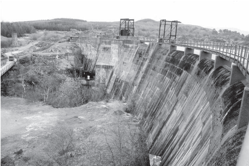
Figure 13.14 Maentwrog Dam in Wales: a case of ASR damage caused by greywacke aggregate.
