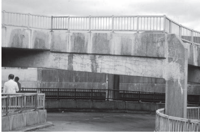
Figure 13.12 Multi-storey car park in Plymouth, Devon: first major structure identified with ASR in the UK.
