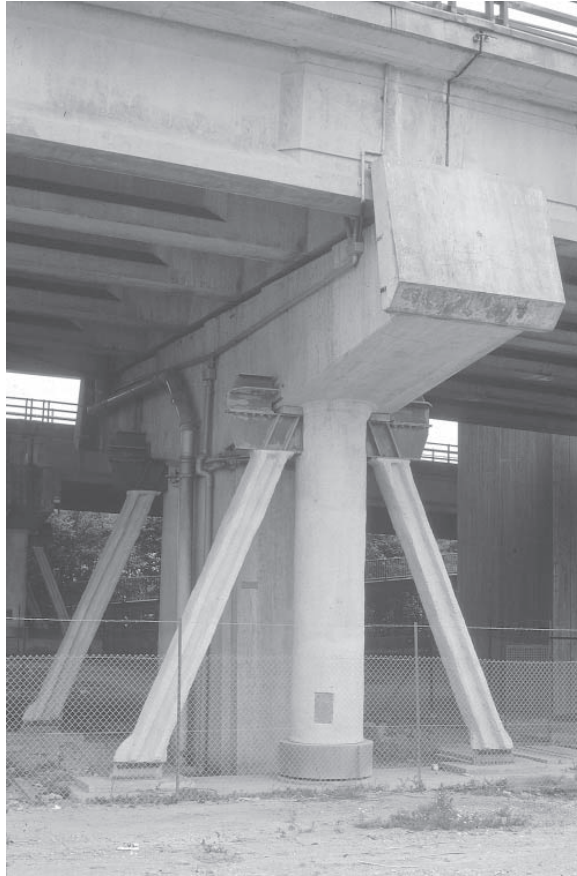
Figure 13.20 Auxiliary support for pier and pile cap affected by ASR: Marsh Mills Viaduct, Plymouth.
