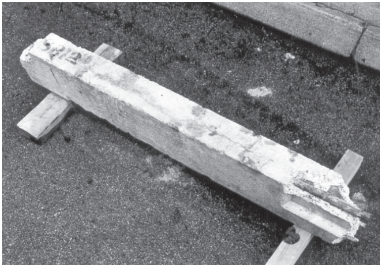
Figure 9.2 Corrosion induced by carbonation of a concrete beam which has resulted in a crack in the concrete cover following the line of the reinforcement.
